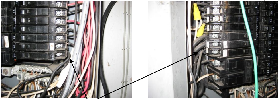
Electrical double tapping.
