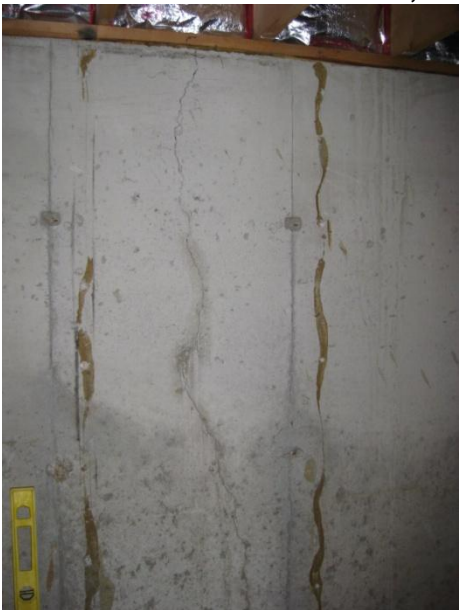
Basement foundation wall north crack.
