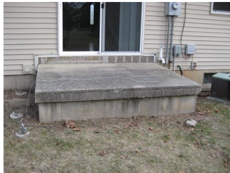
Rear raised slab does not have a step and is a trip hazard.
