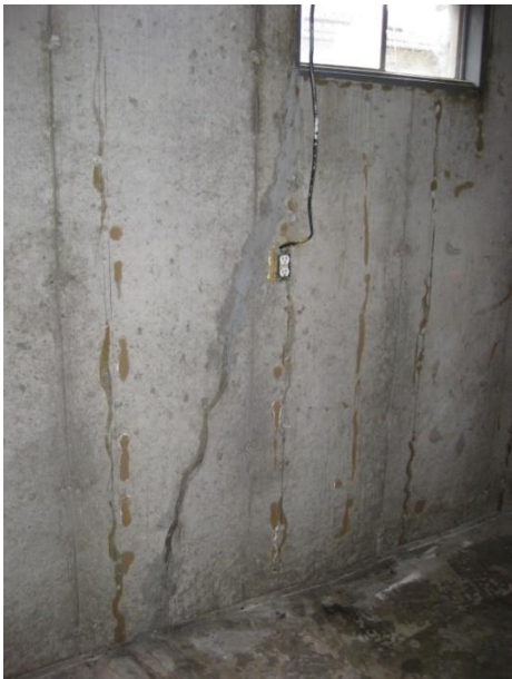
Basement east foundation wall crack.
