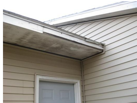
Gutters/downspouts missing on back of garage.
