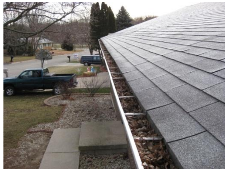
Gutters are full of debris.
